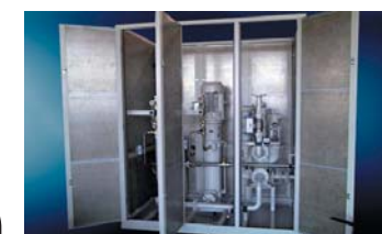
High pressure booster station
